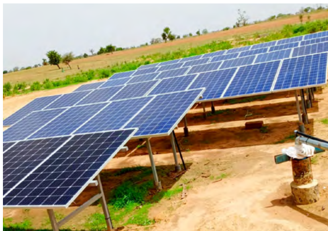
Picture 2: Solar pumping system for irrigating fodder
