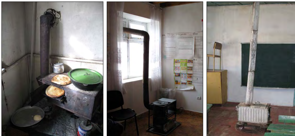
Three examples of chimneys going directly to the outside and removing all hot smoke gasses.
