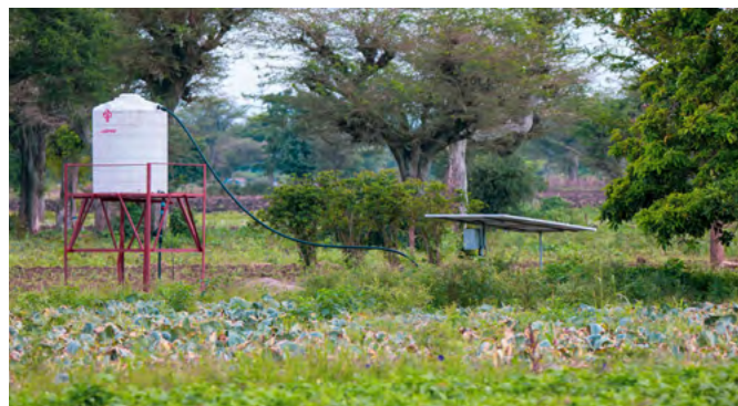
Picture 2: Water Tank, Solar Panels and Water Pump
