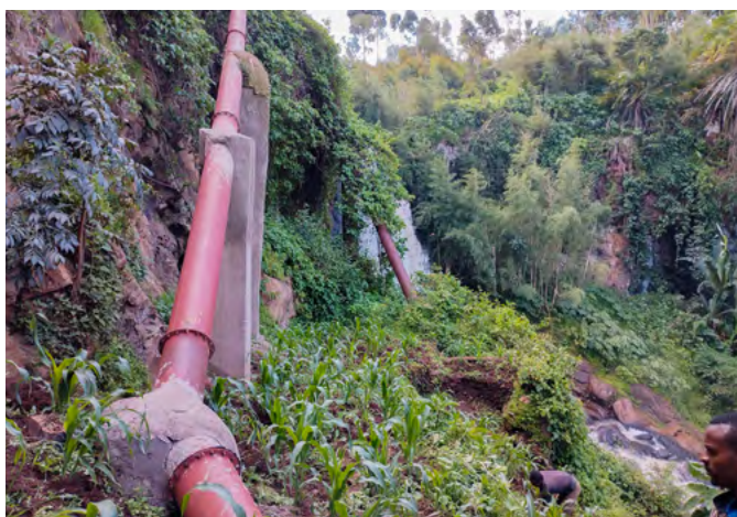
Picture 1: Penstock – MHP Gobecho site
