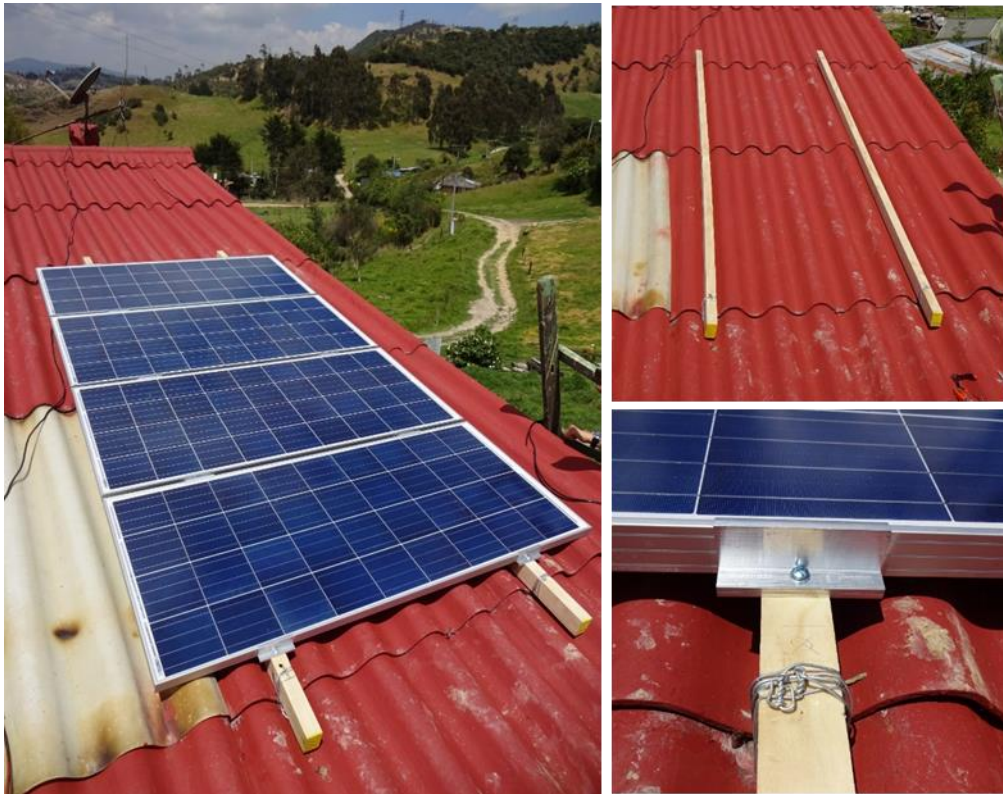
Fig. 5: Provisory fixation of the panels on the roof with a wooden structure
