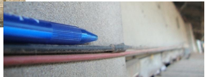
Wire used to connect to a 20 m distanced house (pen diameter is 9 mm)
