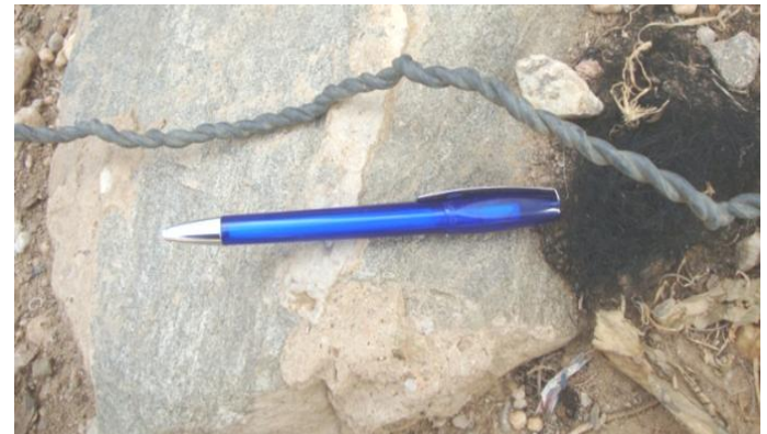
Wire used to connect to a 400 m distanced house (pen diameter is 9 mm)
