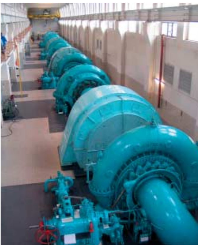
Powerhouse with electro-mechanical equipment from 1932
