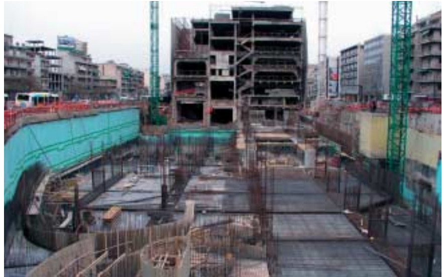
The transfer station Sygrou-Fix is located close to the centre of Athens between two busy roads.
