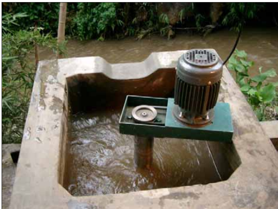
Figure 4-17: Indonesian manufactured unregulated Francis turbine working. Flow: ca. 25l/s; Net head: 3.5m; Power output ca. 450W.
