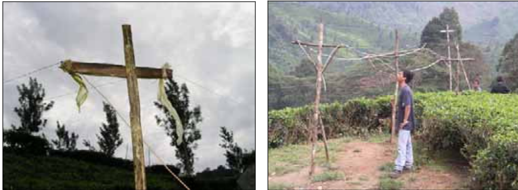
Figure 2-2: Example of bad and dangerous wiring. Indonesia.
