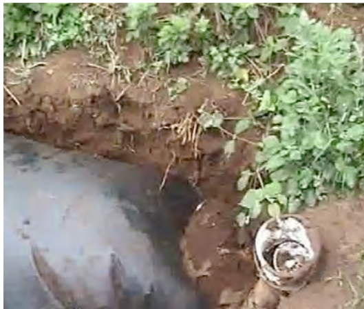
Picture 2: Digester inlet with no trench
