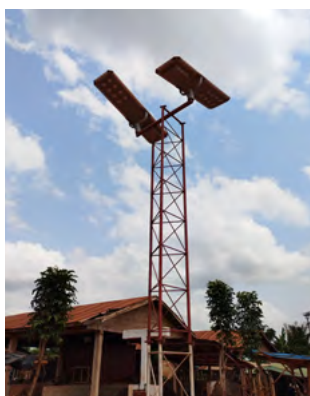
Figure 1: Solar lantern in the local market
