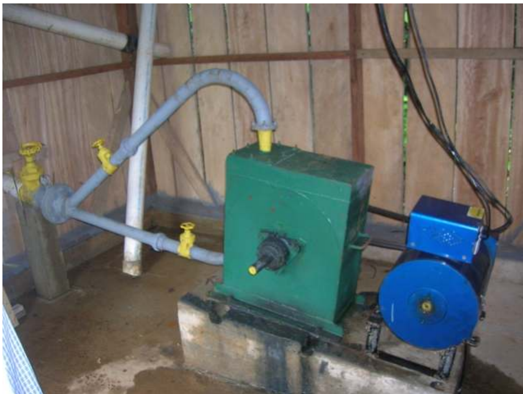
Simple 12 kW Pelton micro hydro turbine with generator
