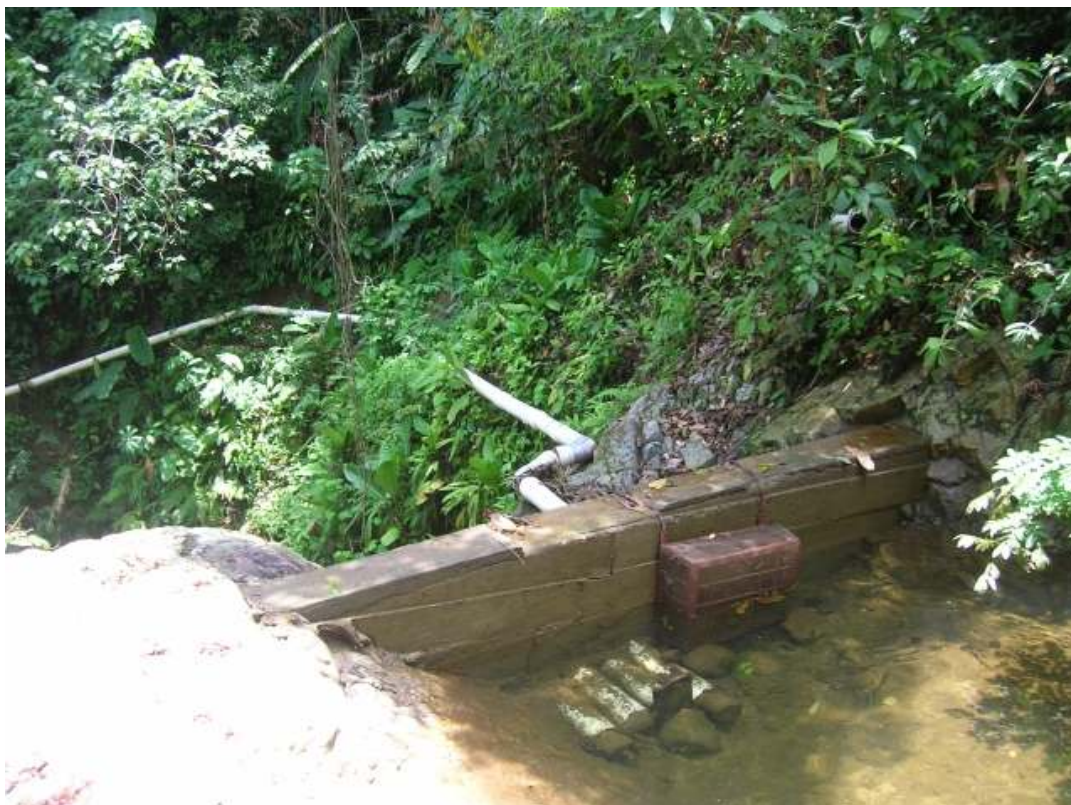
The water intake of the MHP, the 640 m tube has been installed by the local people
