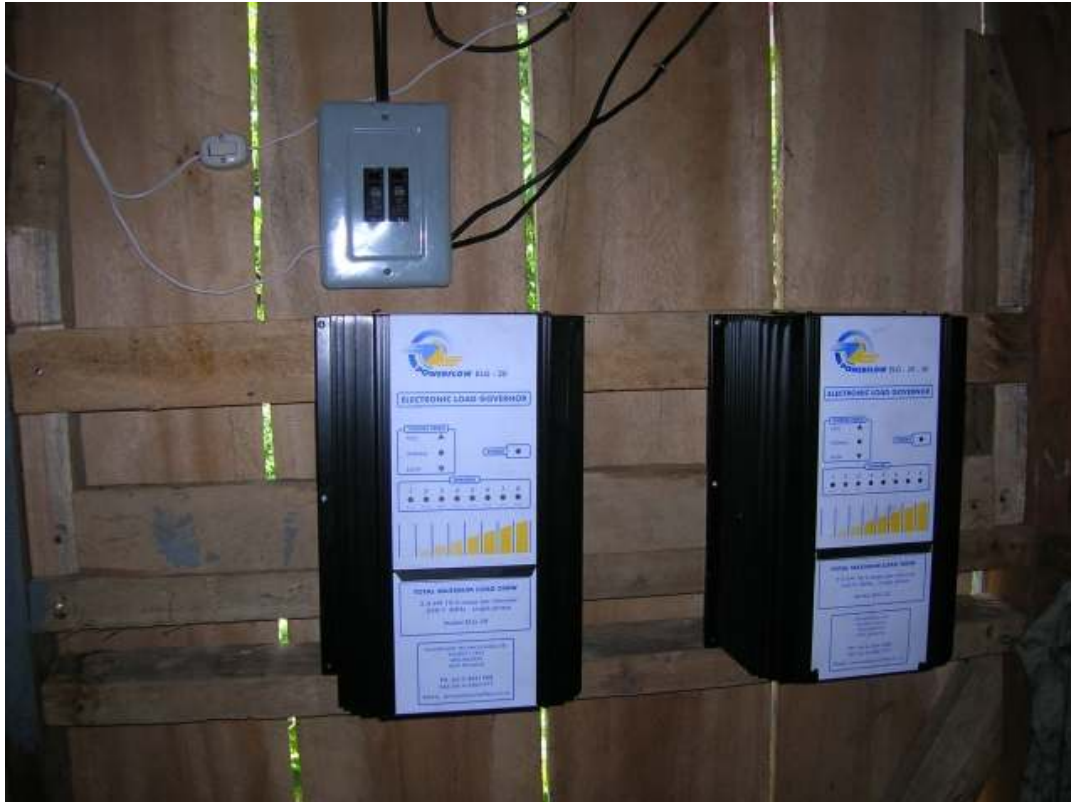
The two load controller are already installed but not connected to the generator
