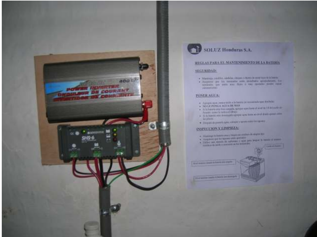
PV controller and AC converter are fixed to the wall, beside a paper of the installing company which explains maintenance of the system
