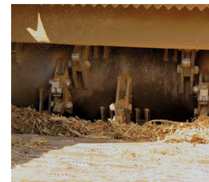
Close-up of Large grinder infeed channel (Courtesy TriCycle, Langebaan)
