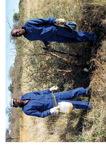
Manual bush pick used here for sickle bush clearing (courtesy Roads Authority of Namibia)
