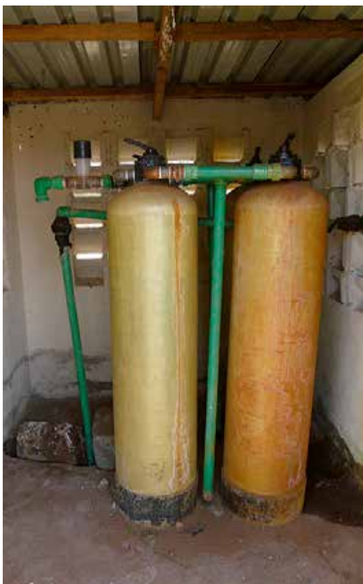
Figure 5.14: Retrofit filter system in Emukutan village, Kenya Source: GIZ / Andreas Hahn, 2015
