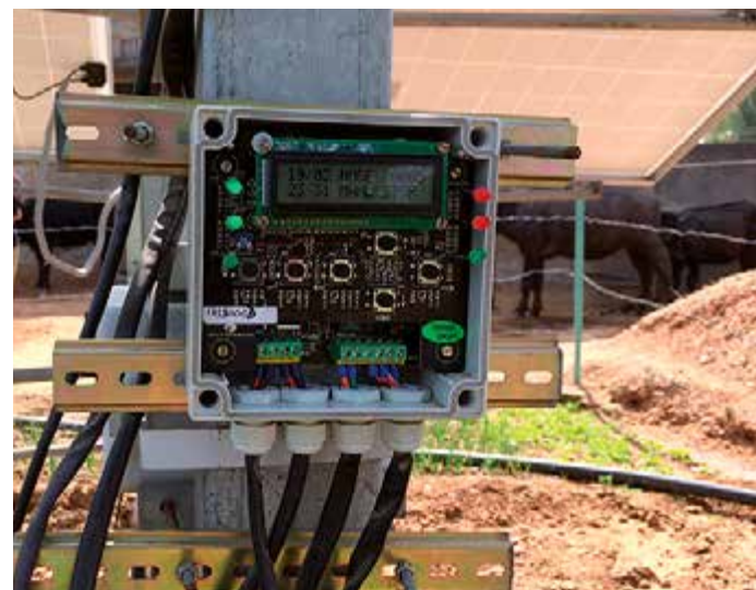
Figure 5.13: Defective tracker control unit in India
