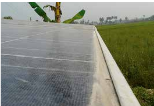
Figure 5.22: Accumulated grime at the lower edge of a PV panel Source: GIZ / Andreas Hahn, 2015
