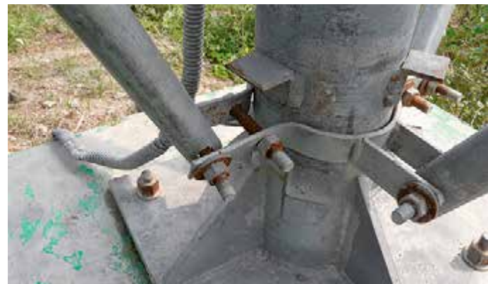
Figure 5.20: Galvanic corrosion of a manual tracking system in India Source: GIZ / Andreas Hahn, 2015
