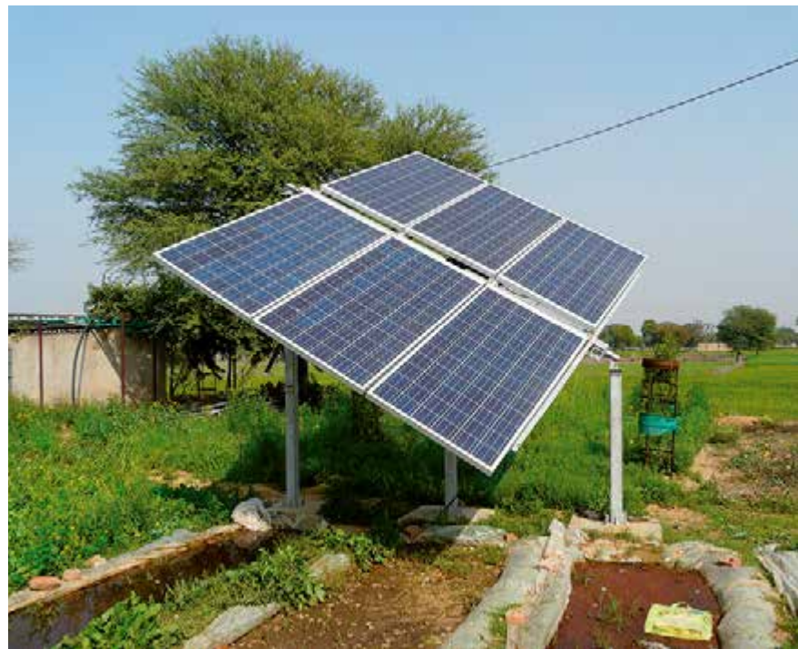
Figure 5.9: Example of an annually operated one-axis solar tracker mounted on concrete foundation in Rajasthan, India
