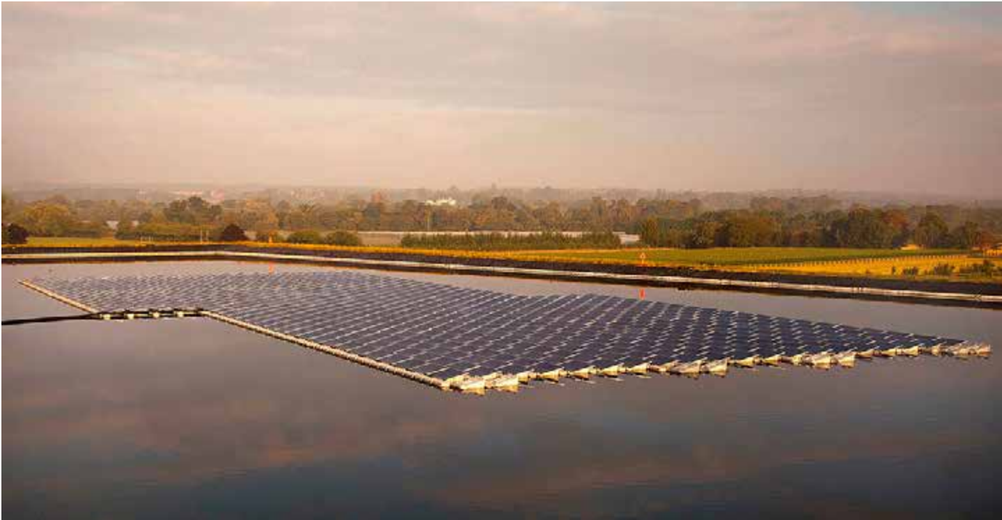
Figure 2.6: Floating photovoltaic modules of the patented floating solar solution Hydrelia®. Sheeplands Farm, UK – 200 kWp
