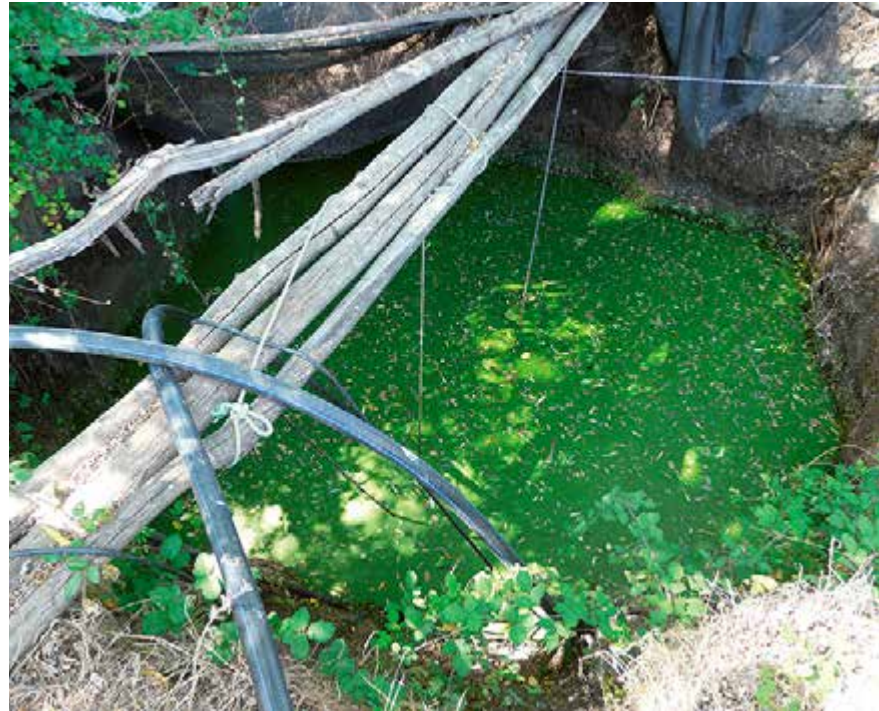
Figure 5.10: Example of difficult conditions for solar water pumps installed in a dug well
