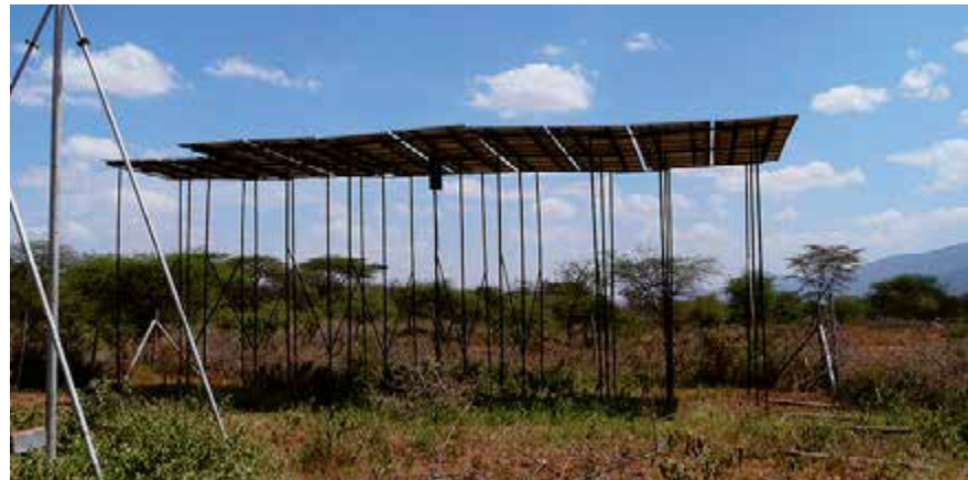
Figure 5.15: Horizontal installation of panels limits self-cleaning of solar generator
