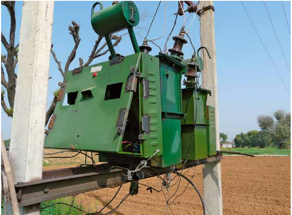
Figure 8.6: Example of an unreliable grid connection in Rajasthan, India
