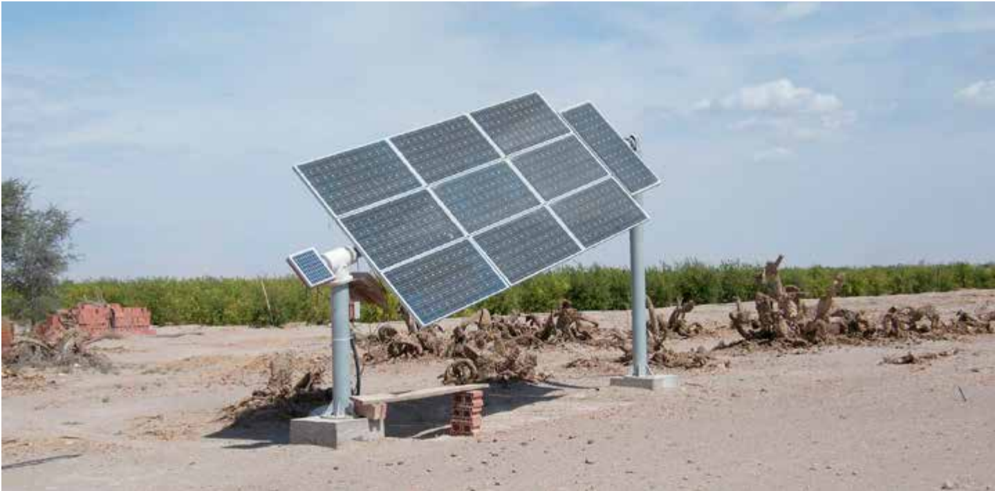
Figure 2.3: A SPIS project in Northern Chile, carried out in cooperation with the farmer and the ministry of energy. The tilted one-axis tracker generates 1kW for a groundwater pump that irrigates 2 ha of pomegranate farmland.
