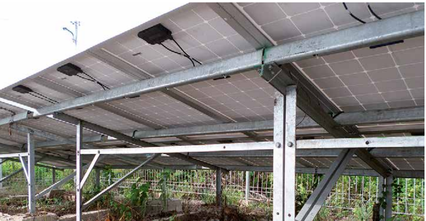
Figure 5.7: Panel and string cables for outdoor applications such as SPIS
