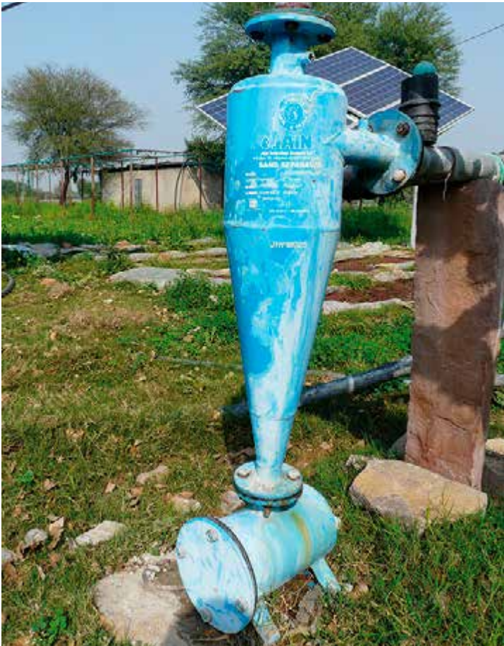
Figure 2.41: Example of a sand separator installation in Rajasthan, India Source: GIZ / Andreas Hahn, 2015
