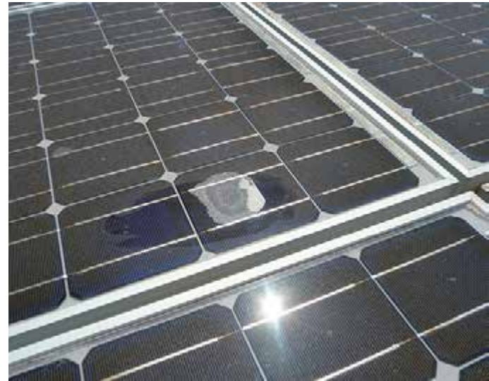
Figure 5.12: First signs of delamination due to humidity ingress
