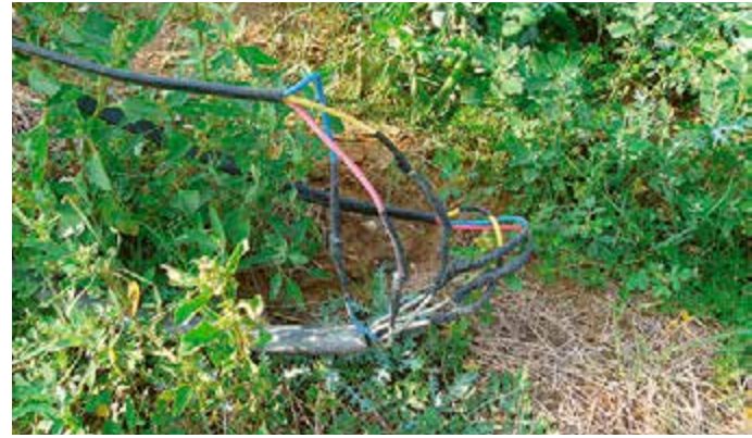
Figure 5.19: Example of a dangerous cable connection Source: GIZ / Andreas Hahn, 2015
