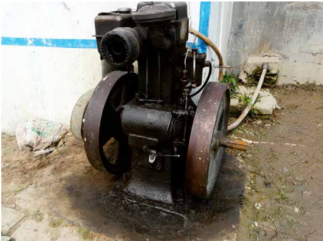
Figure 5.5: Example of a diesel generator causing groundwater and soil contamination in Bihar, India
