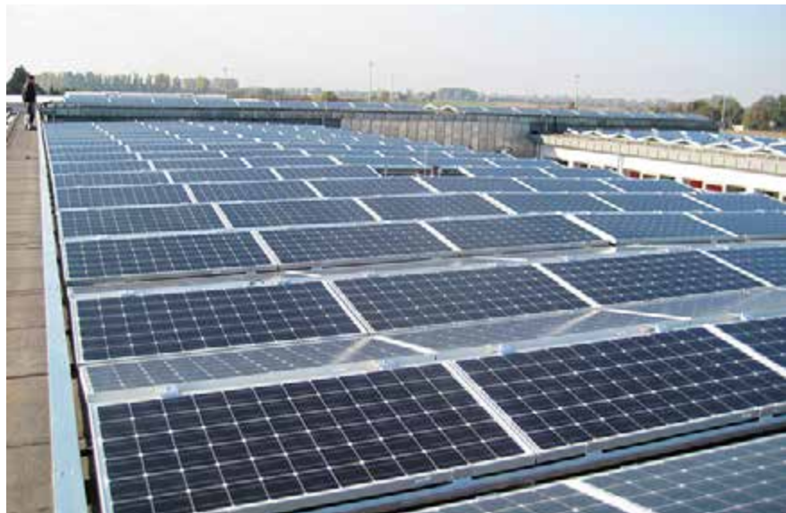
Figure 8.7: East/west orientation of PV panels on industrial rooftop Source: photovoltaikbuero Ternus & Diehl GbR, 2011
