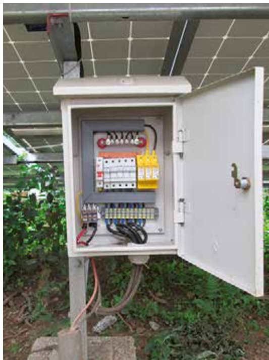
Figure 5.8: Example and string cables for outdoor applications such as SPIS Source: GIZ / Robert Schultz, 2014
