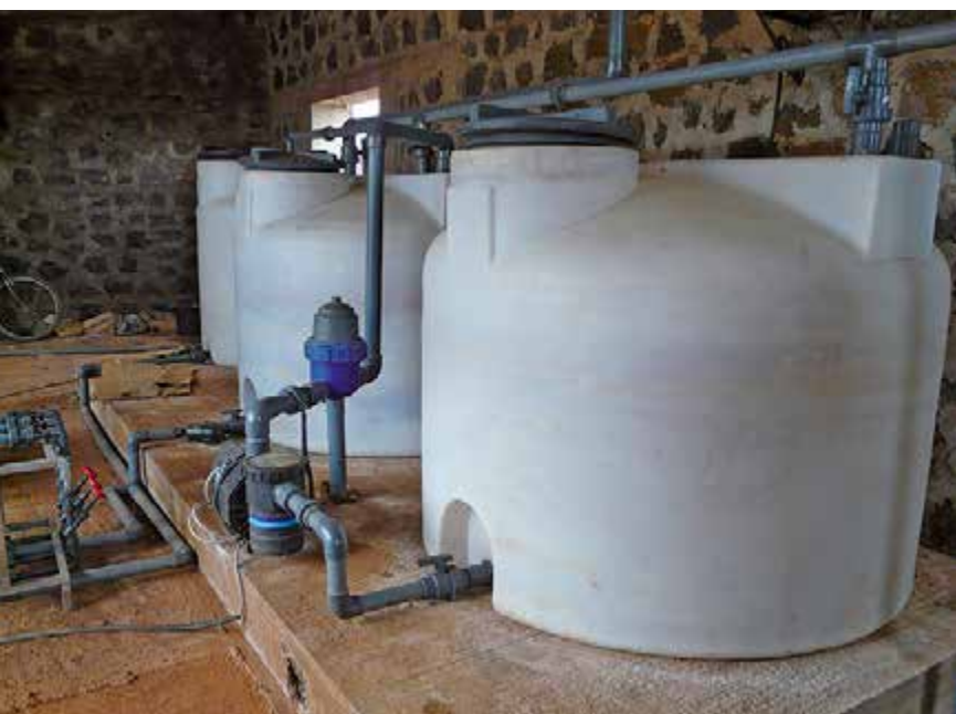
Figure 2.46: Fertigation system at Ain Louh farm in Morocco Source: GIZ / Jan Sass, 2014
