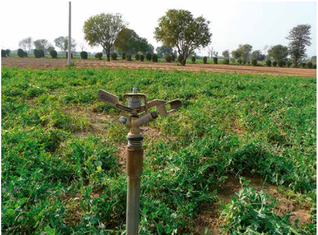
Figure 3.5: Standard impact sprinkler used in combination with conventional and PV pumping in Bihar, India
