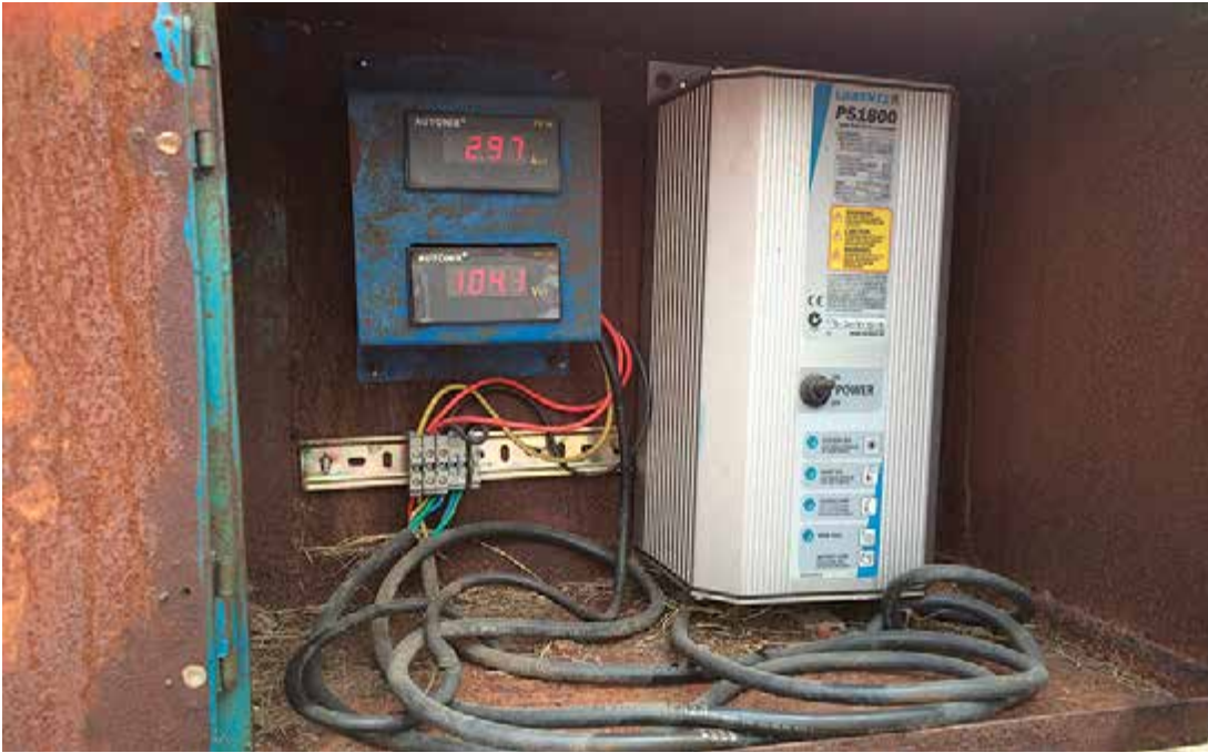
Figure 5.21: Limited heat dissipation capability of corroded controller housing Source: GIZ / Andreas Hahn, 2015
