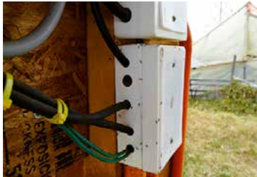
Figure 5.17: Unsealed junction box in Chile inhabited by ants Source: GIZ / Andreas Hahn, 2015
