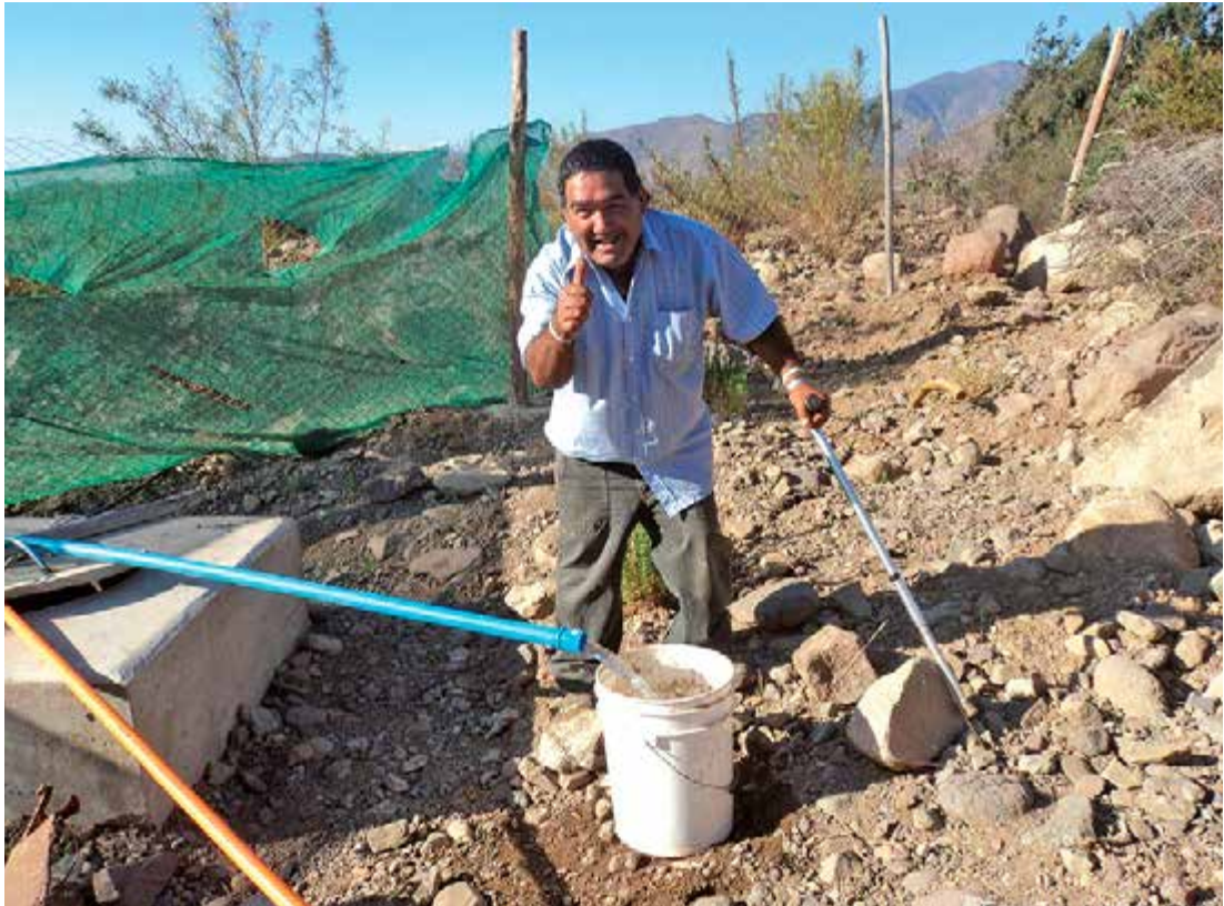
Figure 7.1: Water supply with a solar powered pump in Chile
