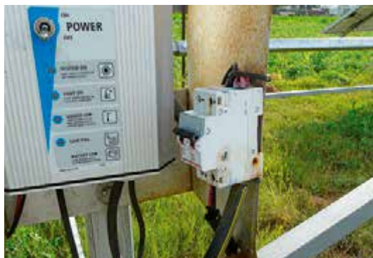
Figure 5.18: Non water-proof circuit breaker in India Source: GIZ / Andreas Hahn, 2015
