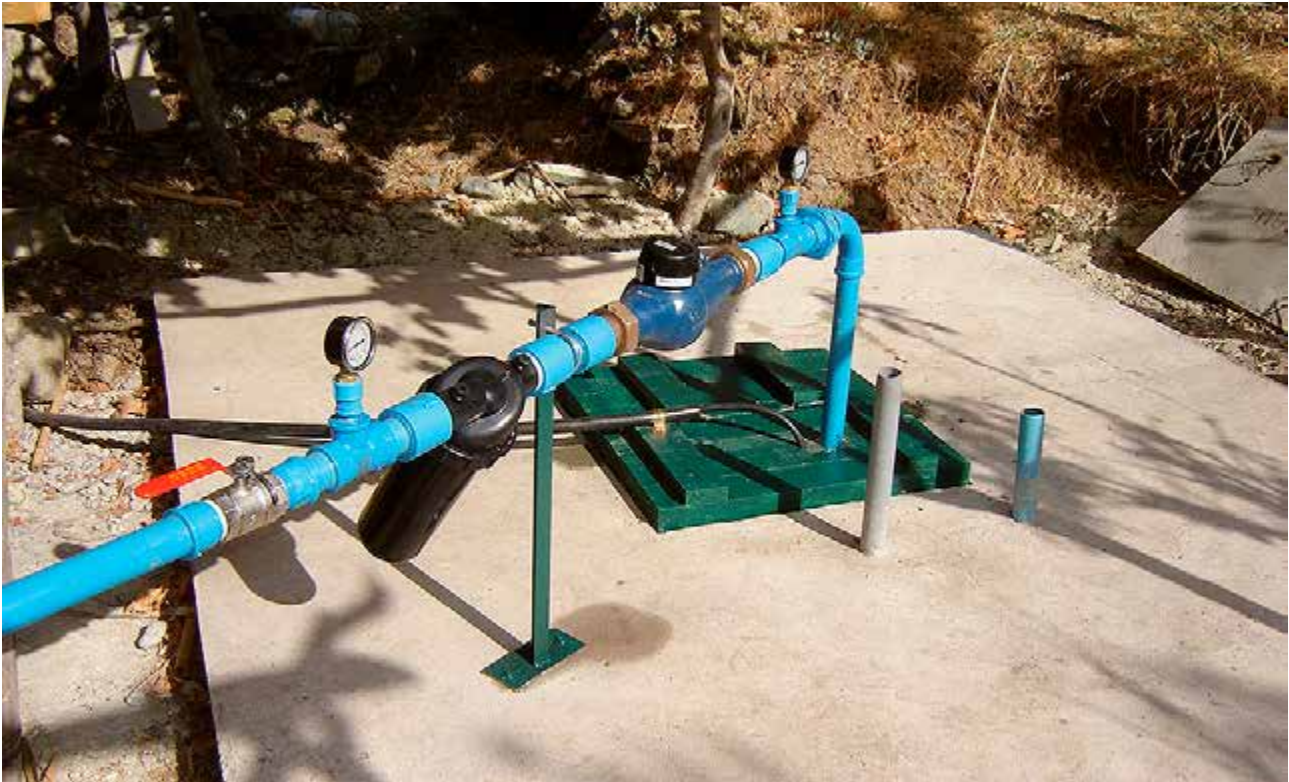
Figure 2.21: Basic monitoring system, installed on site
