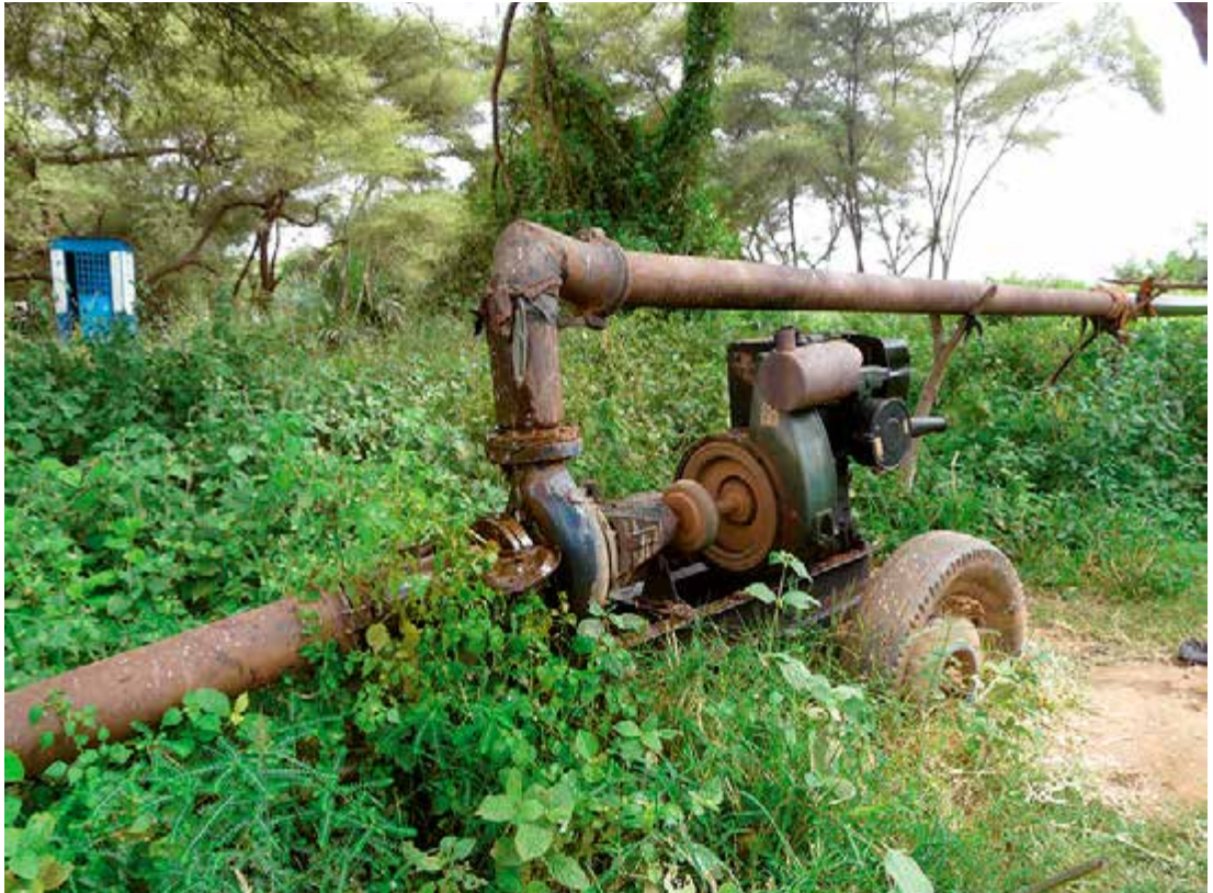
Figure 3.4: Example of an average, maintenance-demanding diesel pump set
