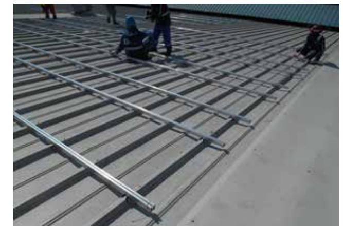
Figure 204: Support structure installation with lines to mark the edges of the profiles and tools for distance control
