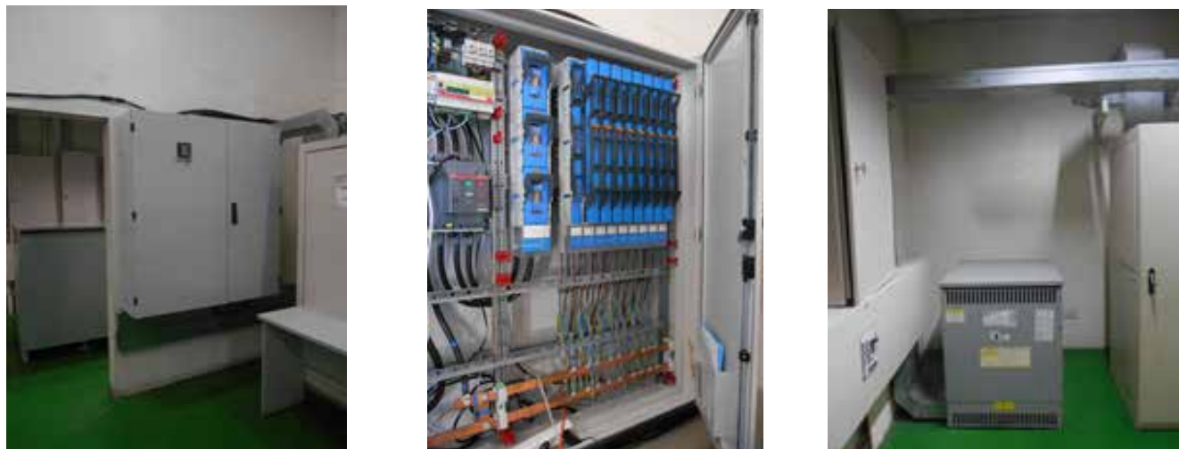
Figure 154: AC connection unit for a 250kWp solar power system with a matching transformer
