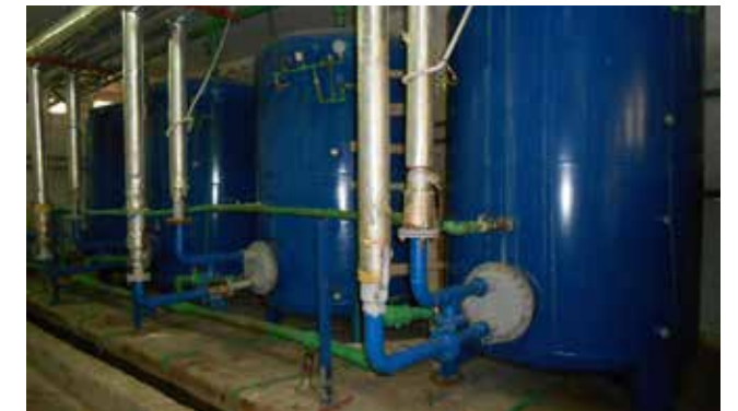
Figure 74: Complex hydraulic domestic hot water system in a tourist hotel
