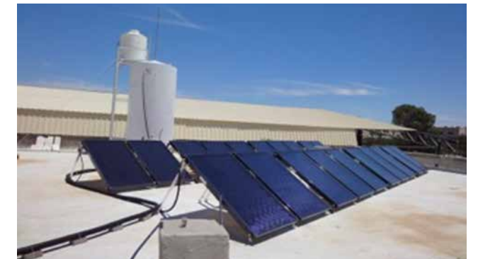
Figure 12: Solar power and solar thermal systems
