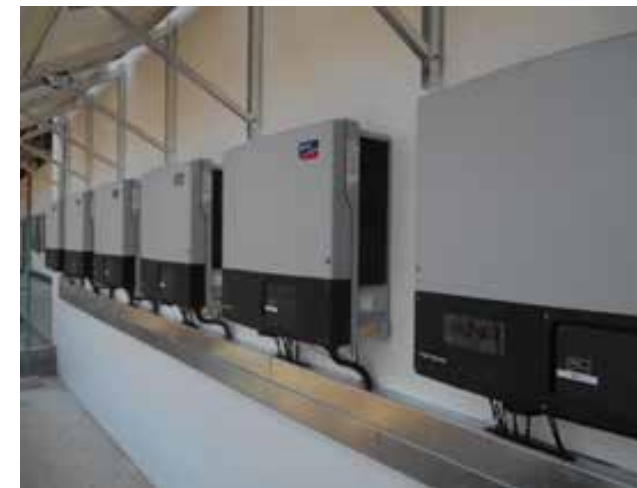
Figure 17: Inverters in a solar power system
