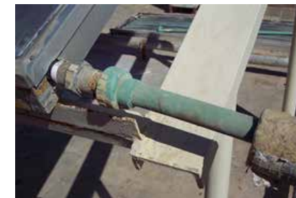
Figure 277: Wrong piping material for hot water or solar installation
