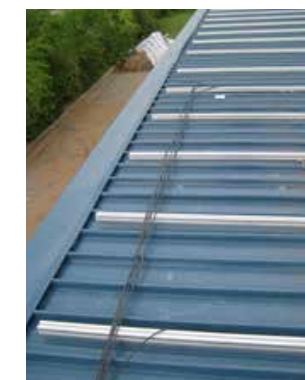
Figure 212: Prepare DC wiring within the module area and solar connector with appropriate crimping tools.
