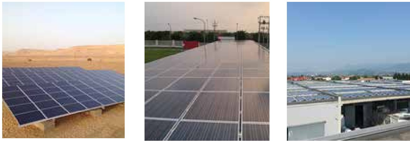
Figure 80: Solar power installations
