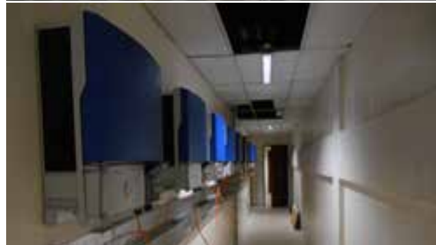
Figure 207: Placement of inverters
