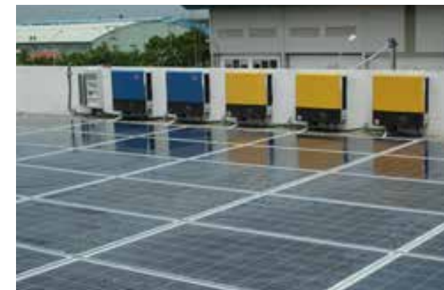
Figure 183: Standard inverters for grid connection
