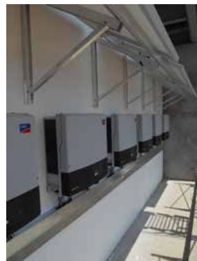
Figure 208: Inverter installation under a solar panel roof for shading
