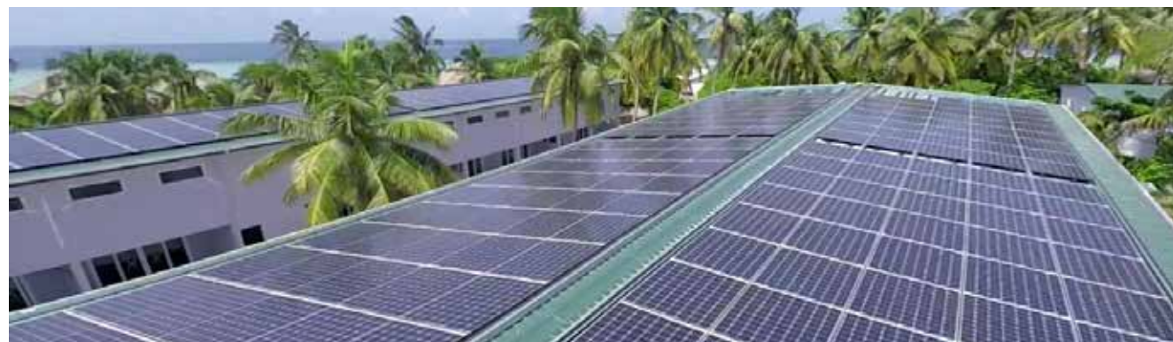
Figure 64: Solar system as a crown on top of a high-rise hotel
