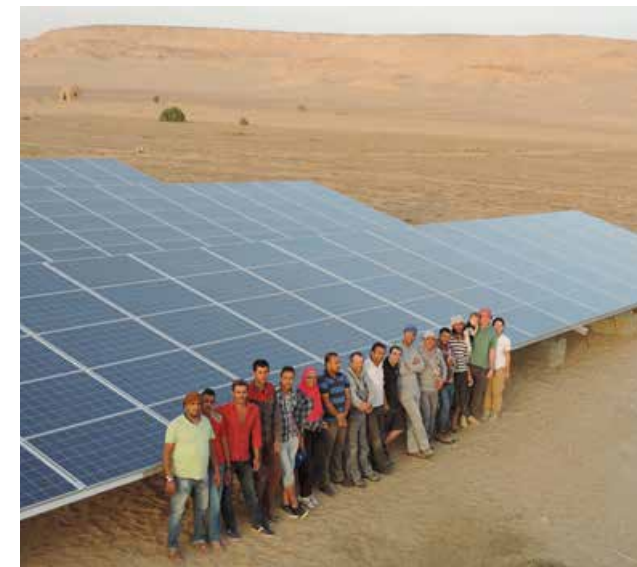
Figure 220: Finished solar power system
