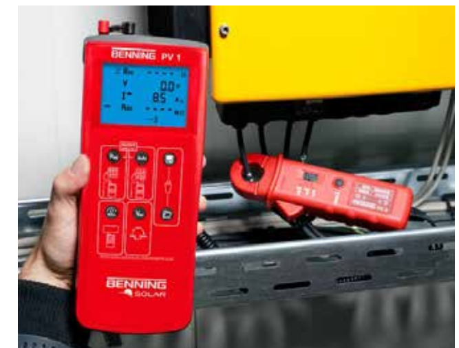
Figure 219: Solar tester to create a start-up and string protocol
