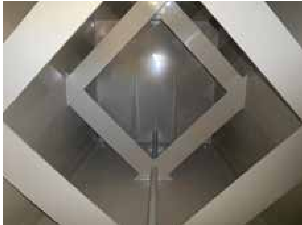
Figure 282: Qualified storage tanks with multi layer coating or anti corrosive materials and separated circles can protect from internal destruction
