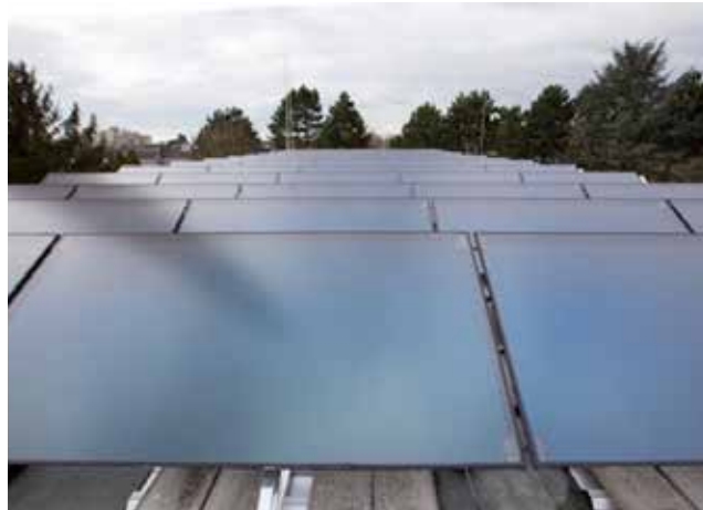
Figure 36: Solar thermal collector
