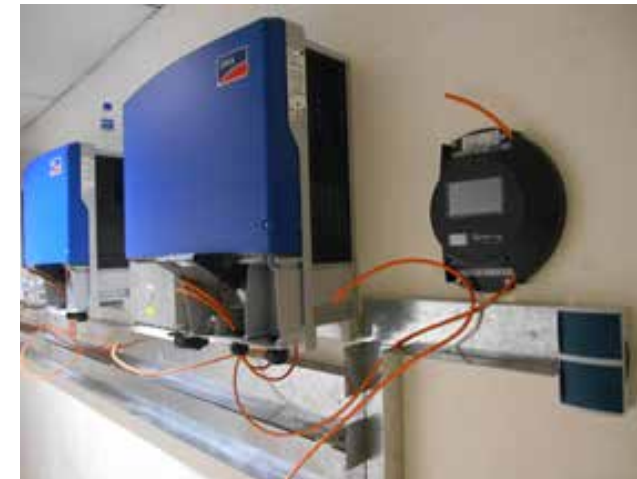
Figure 216: Data wiring of inverters and control device (SolarLog)
