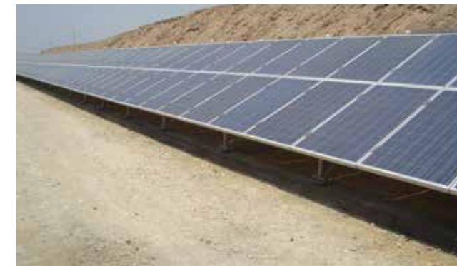
Figure 66: Open area solar power system
