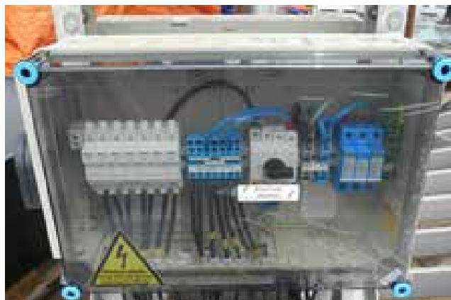
Figure 180: String combiner box in a solar power system
