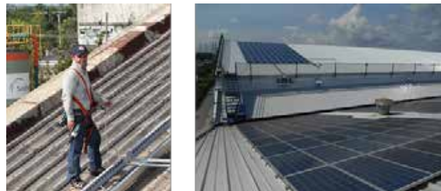
201: Personal safety equipment with a lifeline and a safety net, surrounding the installation area.
