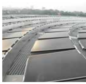
Figure 160: Installation with thin-film modules
