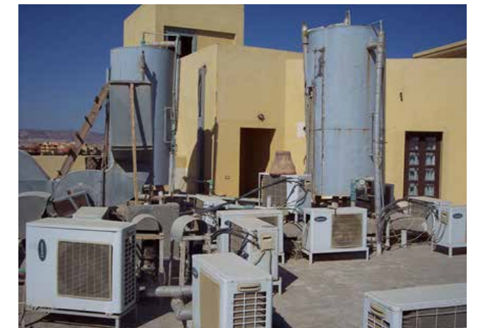
Figure 280: Defect storage tanks and electric heaters.
