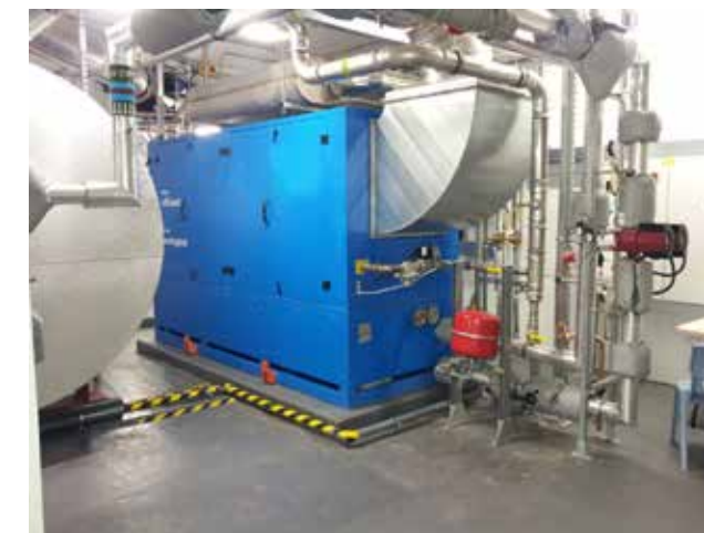
Figure 100: Combined Heat and Power unit
