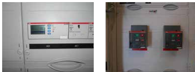
Figure 194: Grid and system protection with monitoring relay and motor switches
