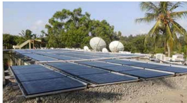
Figure 58: Hidden solar thermal system on an apartment hotel
