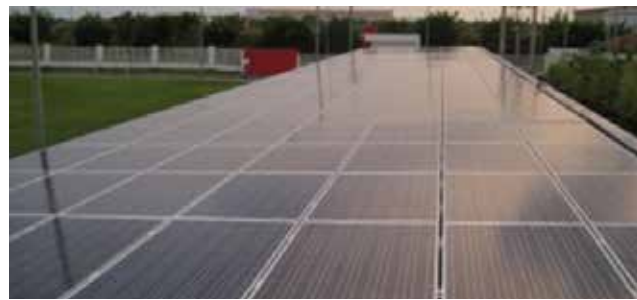
Figure 18: Installed PV modules
