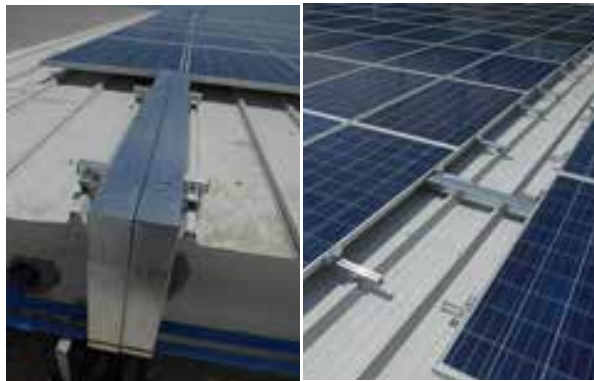
Figure 213: Cable duct for DC wiring on the roof and AC wiring at the inverter
