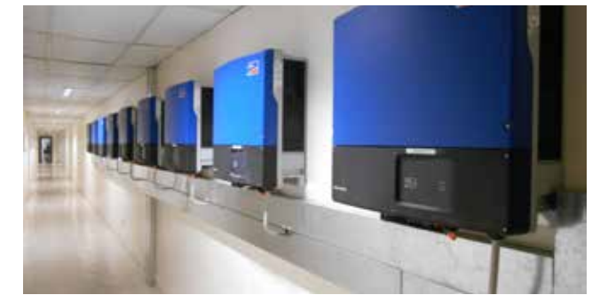
Figure 138: Typical string inverters with strings directly connected to the inverter
