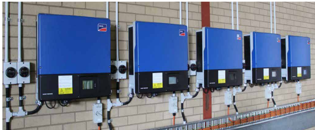
Figure 25: Solar inverter installations
