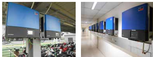
Figure 181: Different inverter installations of outside and inside solar systems
