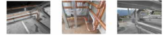
Figure 253: Perfect copper pipework with insulation in aluminium casing
