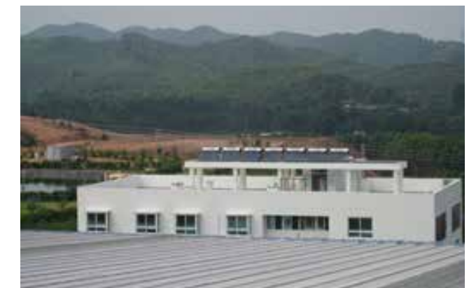
Figure 56: Multi-Solar Water Heater system for smaller hotels
