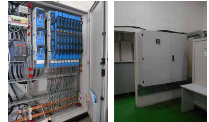
Figure 218: Installed AC connection unit
