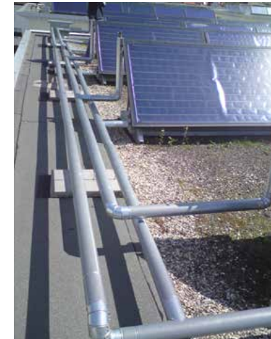
Figure 260: Mineral wool with a metal sheet casing
