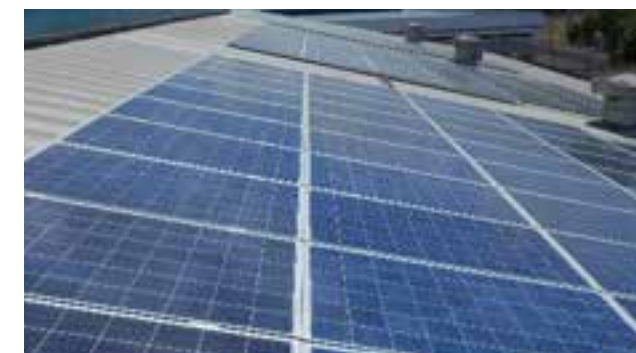
Figure 158: Installations of polycrystalline modules
