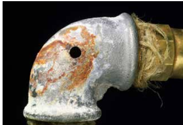
Figure 75: corrosion on pipework through the aggressive water from the sea
