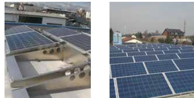
Figure 171: Typical flat roof installations
