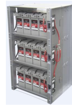
Integrated Battery Rack
