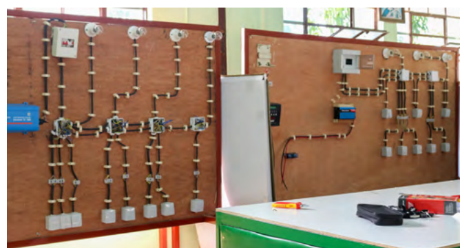
Picture 2: Board set up by students and teachers after receiving the equipment
