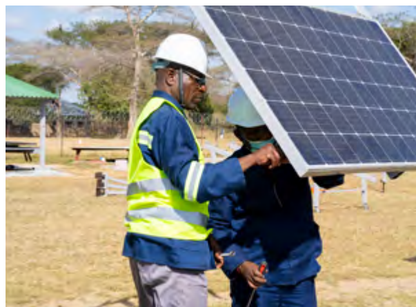
Trainee positioning a solar module during practical assessment of training of trainers by TVETA in Zambia
