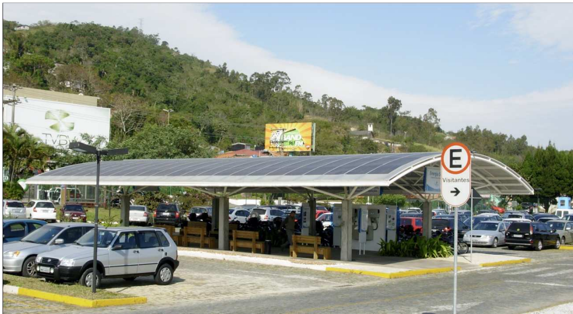
Figure 9: PV system at Eletrosul (2010)
