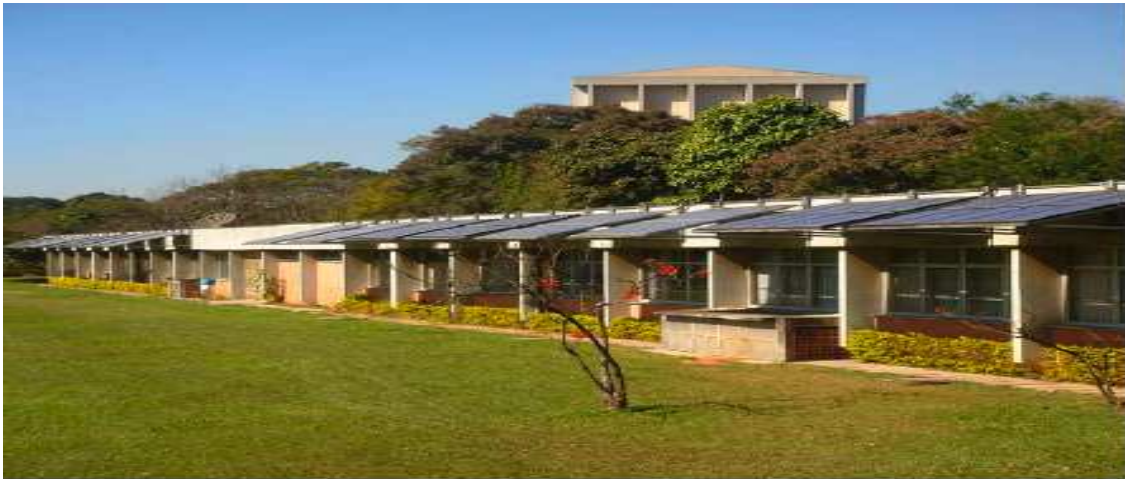
Figure 6; PV system at USP Zilles (2010)
