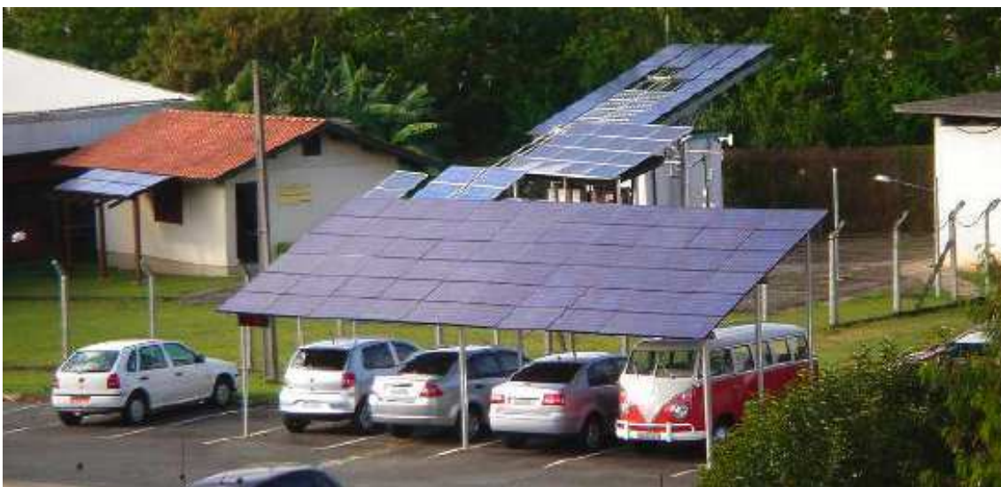
Figure 7: PV system at USP Zilles (2010)
