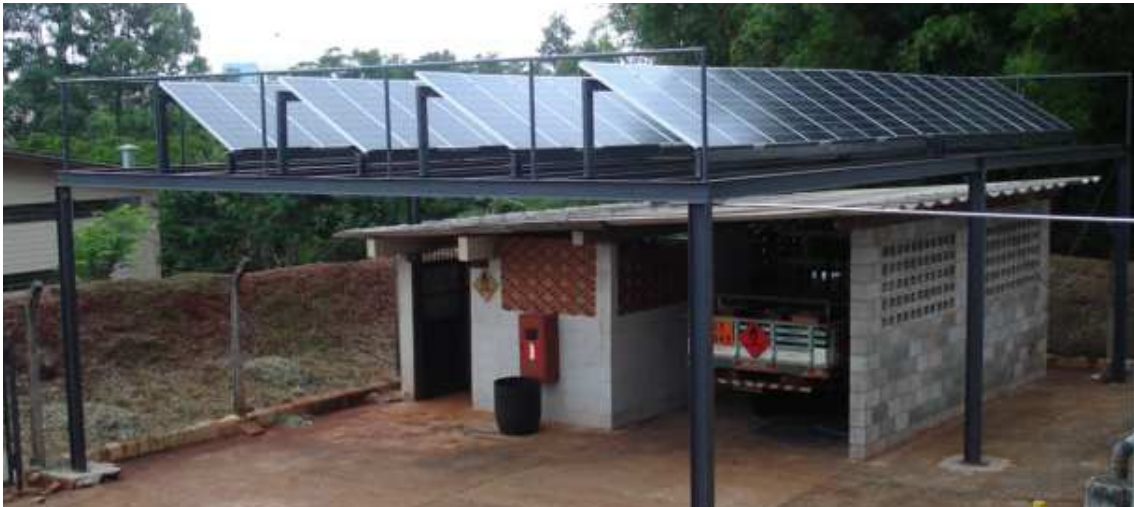
Figure 8: PV system at LH2 (Carmago, 2010)
