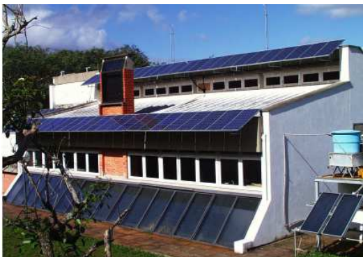
Figure 5: PV system at UFRGS (Dias, 2006)
