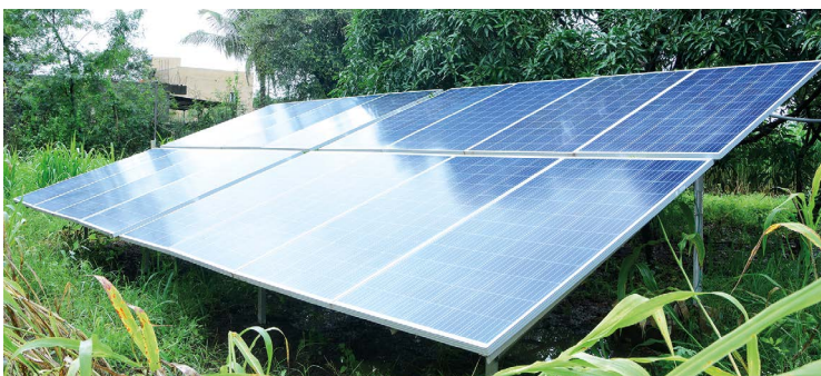
Figure 5.9 Array of solar PV modules (Promethean).
