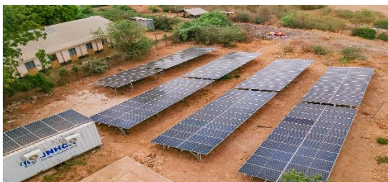
Kaapoka Health Centre in Kakuma, one of the facilities solarized by UNHCR. © GIZ Kenya, 2023
