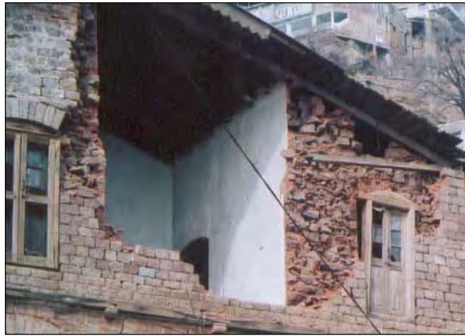
COLLAPSED AND FALLEN AWAY
