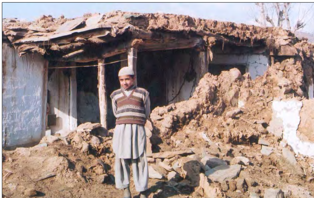
TRADITIONAL HOUSE ~ COLUMNS JUST MANAGE TO KEEP THE HEAVY ROOF UP. WITHOUT THE REMAINING BRACING WALLS, THE STRUCTURE WILL COLLAPSE FURTHER.
