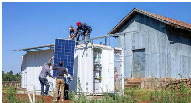
Picture 1: Solar panels powering the solar container
