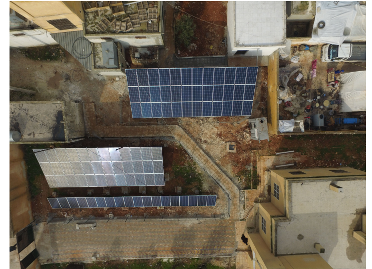
Example of 20 kWp PHC
