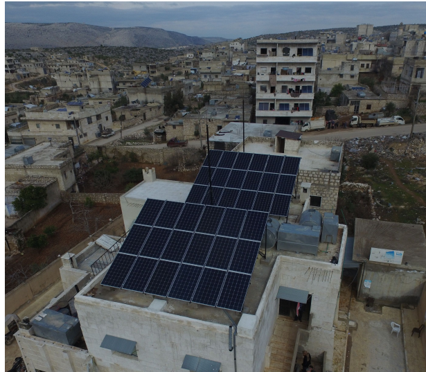
Example of 10 kWp PHC
