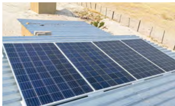
Solar system funded with a credit provided by the SRF in Namibia
