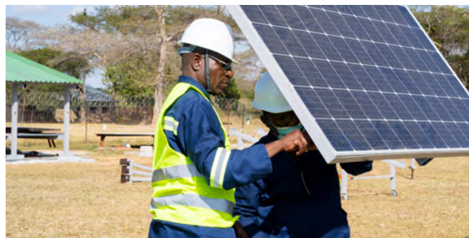
Picture 2: Trainee positioning a solar module during practical assessment of training of trainers by TEVETA
