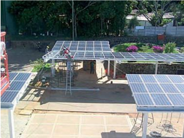
Figure 1: The final solar module is installed on the parking lot of ‘Pituaçu Solar’ (15.03.2012)
