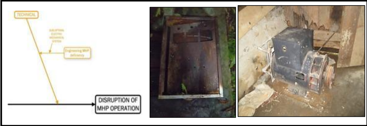
Figure 35 Burnt control panel in Embonatana (left) and broken generator in Lemo Menduruk (right)
