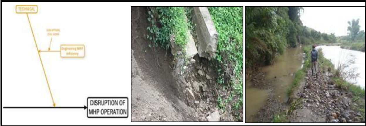
Figure 36 Poor quality of civil works
