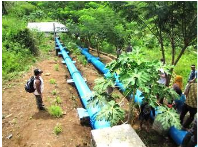
Figure 9 Two penstocks one powerhouse
