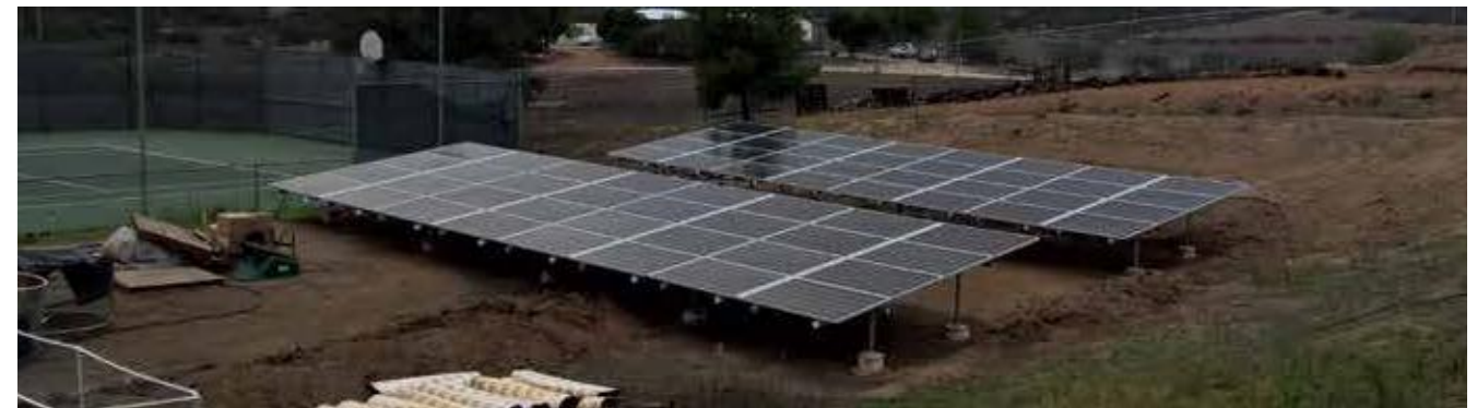
SOLAR POWER FOR RESIDENTIAL SCALE – ALPINE CA. 91901 LOCATION: ALPINE CA. 91901 Estimated lifetime production: 24.8 MWh
