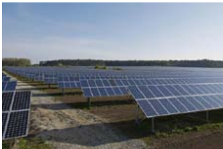
PV POWER PLANT
