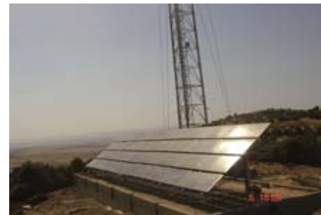
TELECOM POWER SUPPLY
