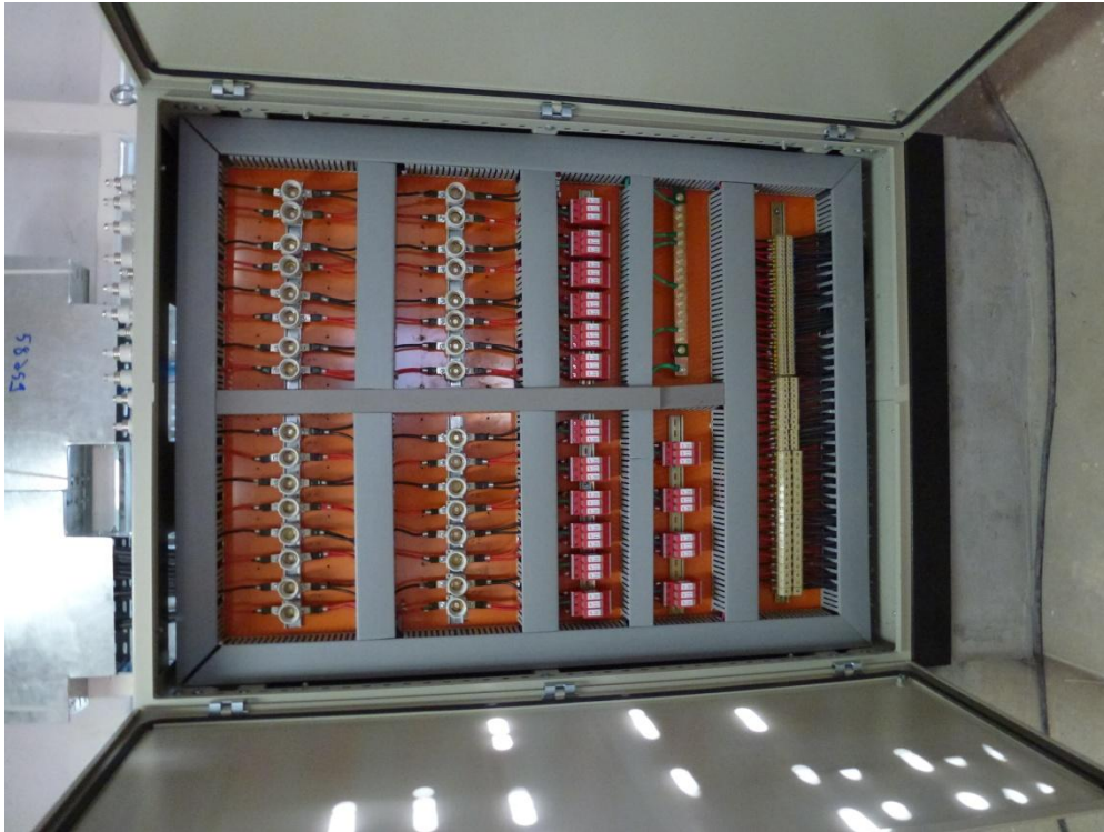
Figure 39: Generator connection box.
