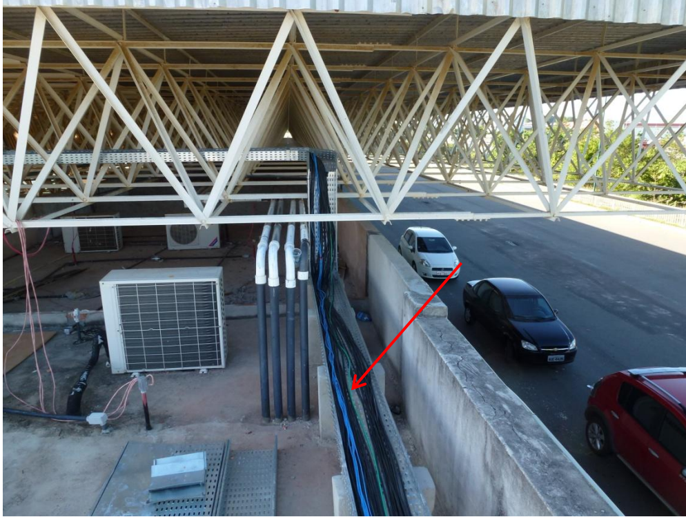
Figure 2: Data cable in same cable tray as power cables.
