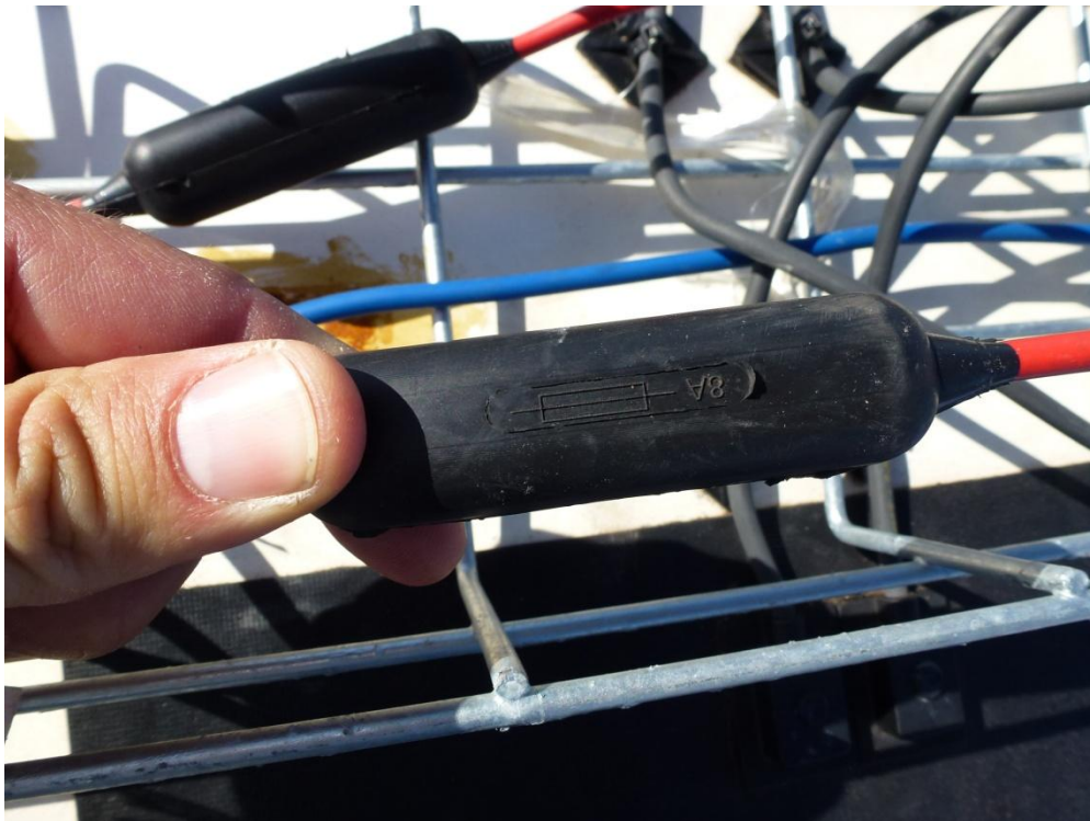
Figure 38: String fuse by Gehrlicher Solar for PVL-144 in Area 4.
