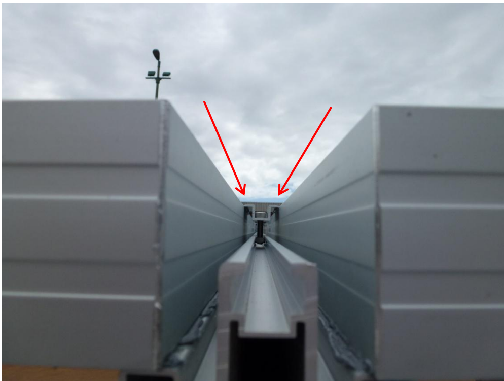
Figure 13: Incorrectly installed module clamp (2).
