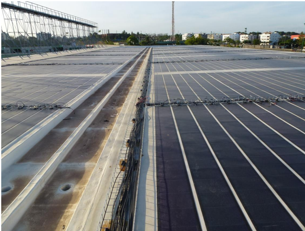
Figure 1: Open cable trays.
