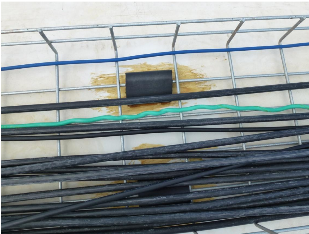
Figure 11: Tightly curled cable for protective earthing.
