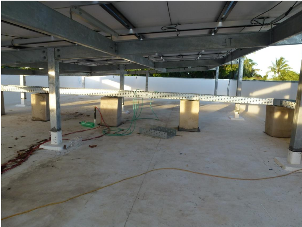
Figure 16: Grounding not connected in Area 2, unidentified red cable, waste.
