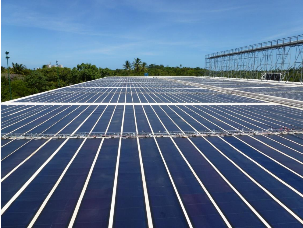
Figure 31: View of Area 3 with PVL-144 modules from Uni-Solar.
