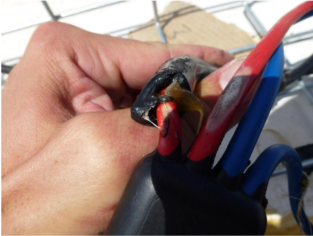
Figure 10: Incorrectly installed cable connection.
