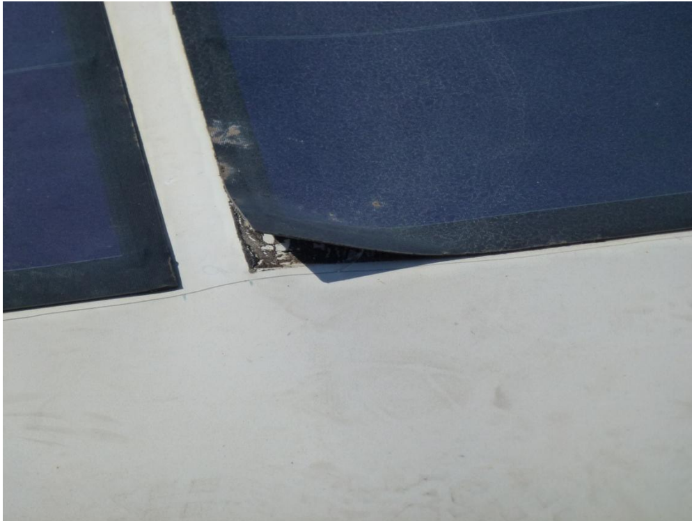
Figure 8: Laminate not completely attached to the roof.
