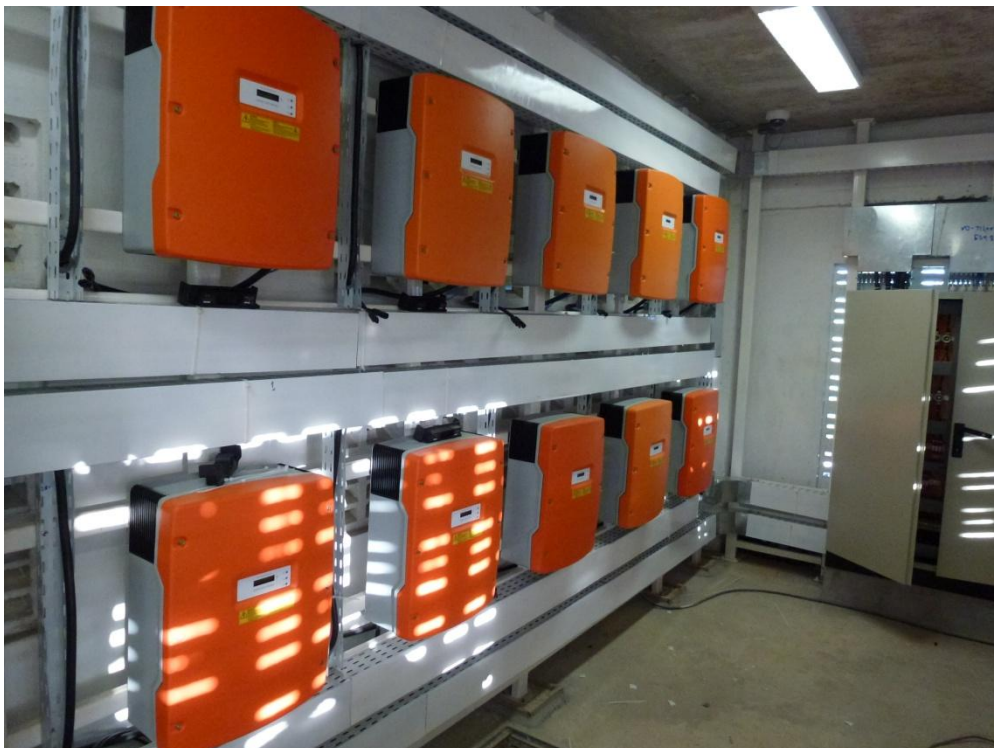
Figure 40: Inverters installed in inverter room.
