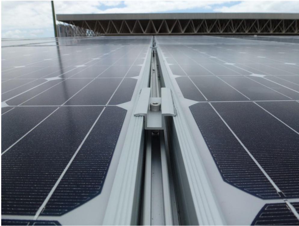
Figure 12: Incorrectly installed module clamp (1).
