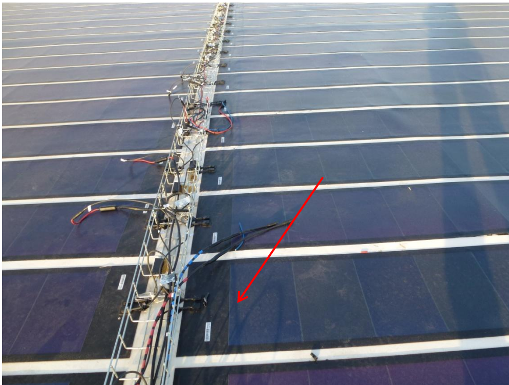
Figure 3: Strings not connected, shading of modules by cable tray.
