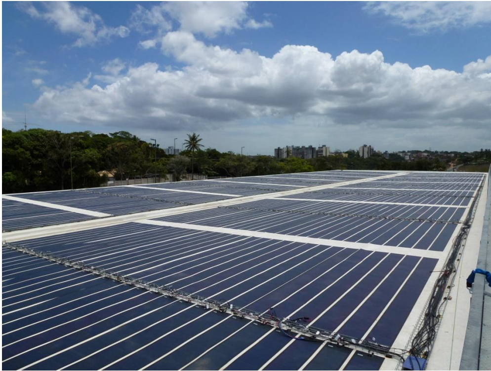
Figure 33: View of Area 4 with PVL-144 modules from Uni-Solar.
