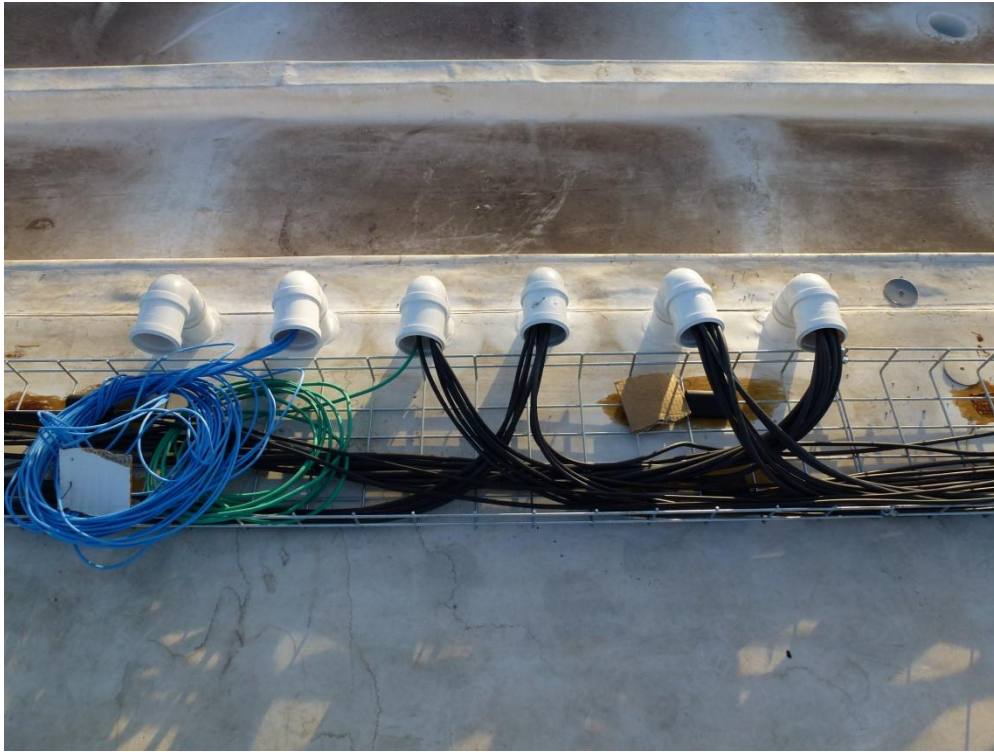
Figure 6: Cable conduit of non UV resistant material, grounding not connected.
