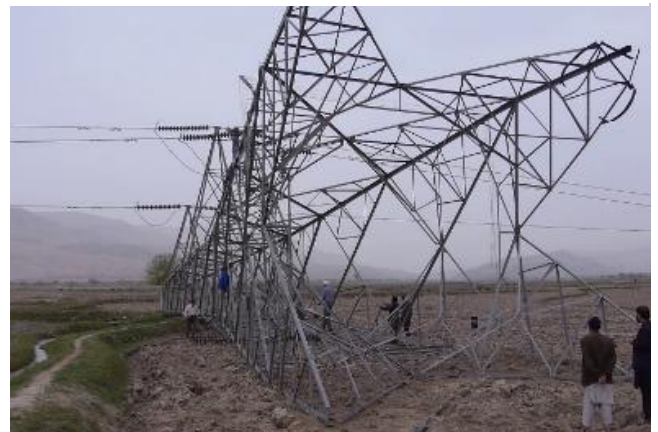
Figure 6 A pylon downed during fieldwork. DABS official image.
